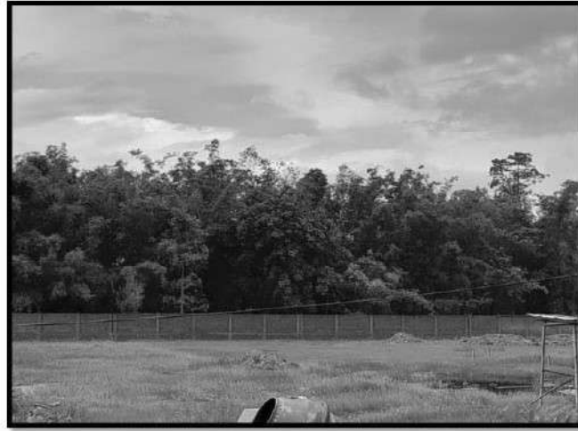
Fig. 2 Photograph showing Ongoing construction of ITI at Sootea Town (Govt. of Assam funding)
