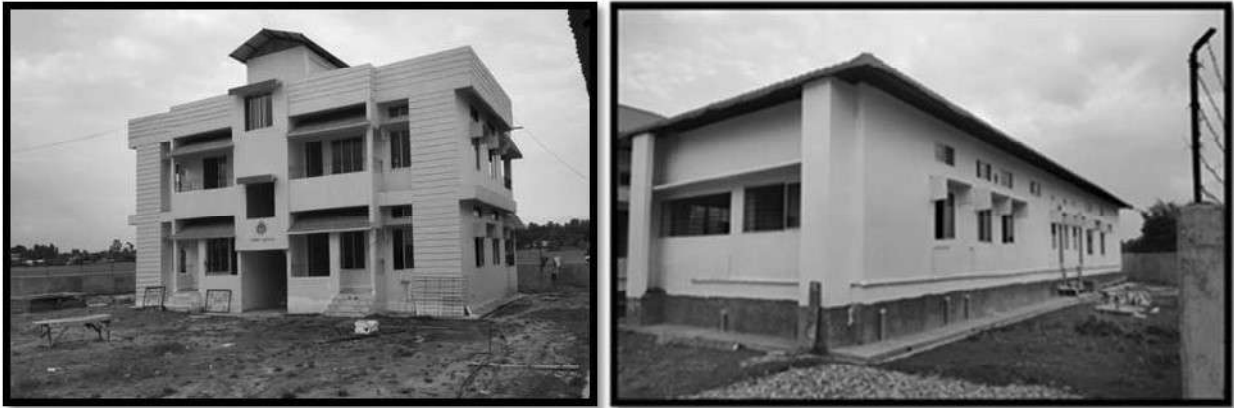
Fig. 4 Photograph showing Ongoing construction of 30-bedded Model Hospital, Sootea Town (NHM funding. Project Cost: Rs. 6.00 (six) Crores)
